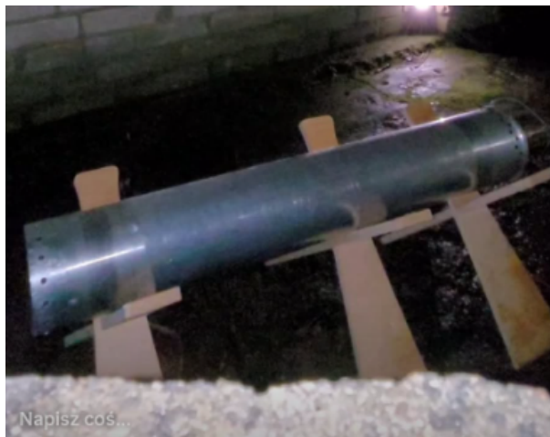
Figure 4.22: Combustion chamber during hydro-test.
